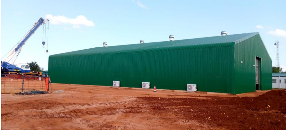
Figure 1 - Equipment Assembly Facility
